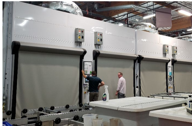
Climate controlled grow chambers used by a large indoor facility.
