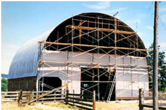
A barn at the Rice Ranch under refabrication in 1999. (Rice Family Photo)
